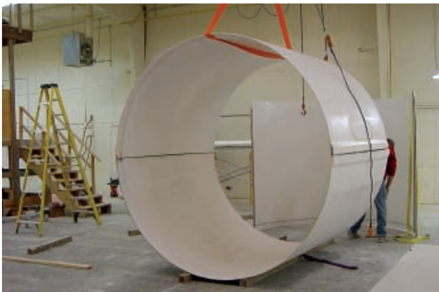
ArmorGRIP® panels by Insituform are assembled to rehabilitate a large sewer line.
